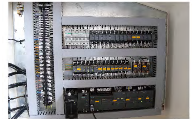
电器箱 Electrical cabinet
