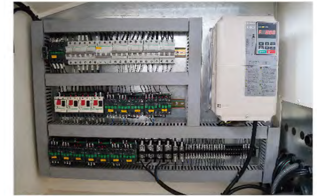
电器箱 Electrical cabinet
