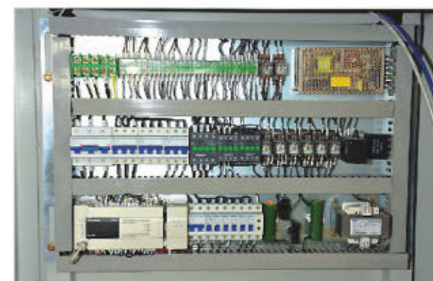
电器箱 Electrical cabinet
