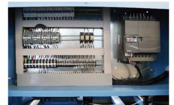
▲ 倒轴电气控制系统 Beaming electrical control system
